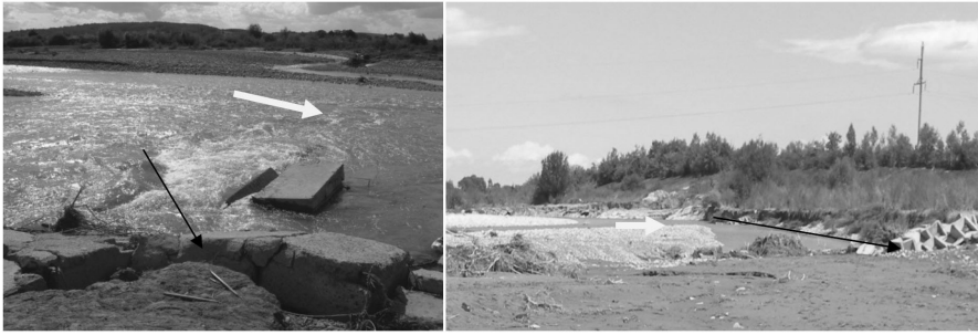
Figure 2. Destroyed diking dams on the right bank of the Bystrytsya Nadvyrnianska River.
