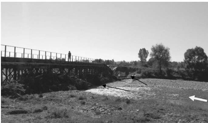
Figure 4. Partially destroyed bridge of the Chechva river near Dovhe Kaluske village
