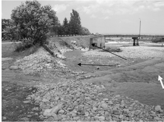
Figure 5. Destroyed the left bank and the road before bridge on Limnytsyu river in Perehinske
